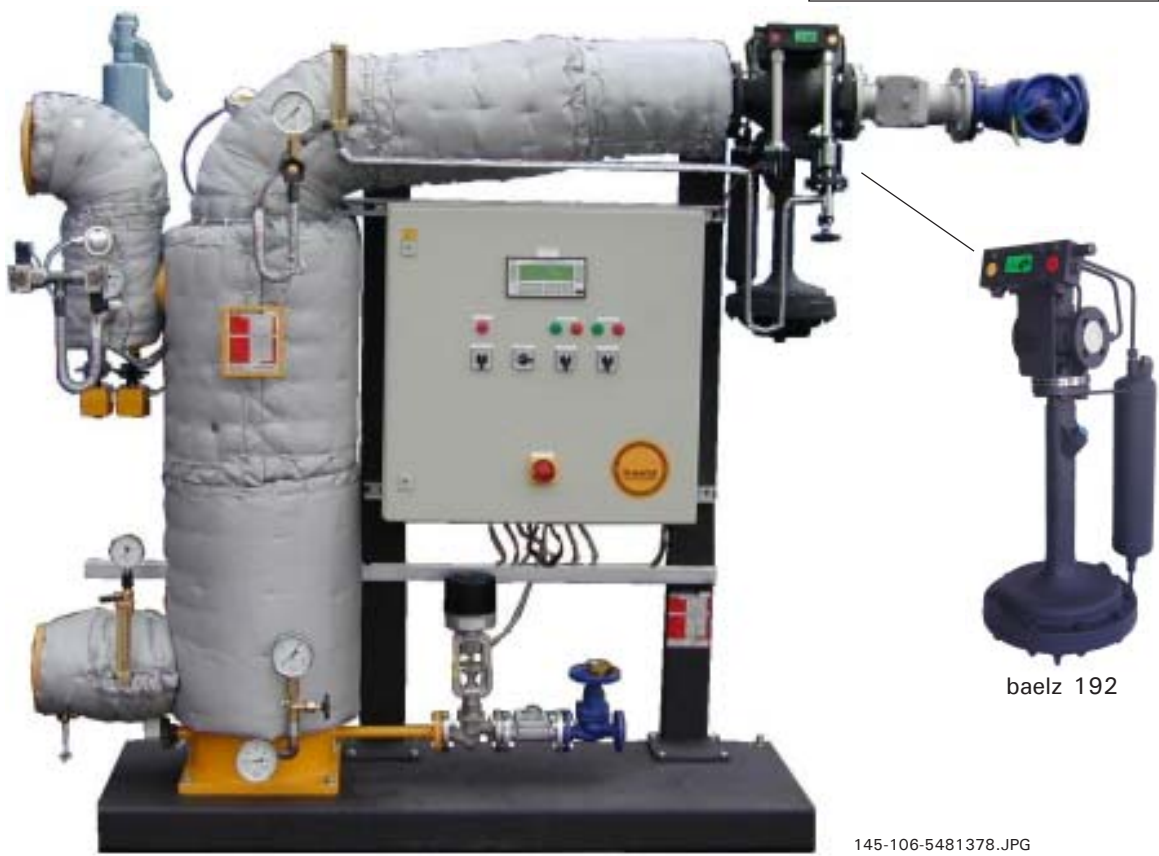
Fig. 22 typical application of the baelz 192 as emergency stop - valve and steam pressure reducing valve ahead of an steam / water heat - exchangers with condensate outlet control
